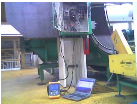
ELELCTRICAL MOTOR ENERGY AUDIT
